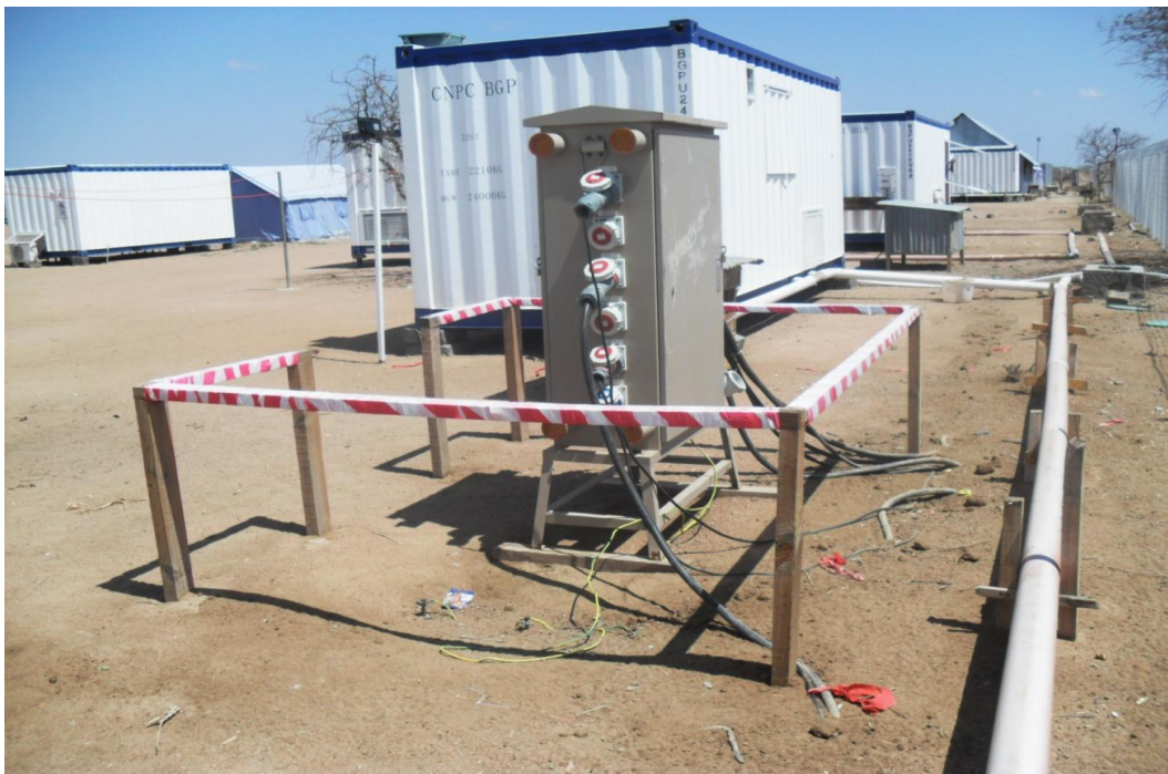
Figure 8: Power Distribution Unit
