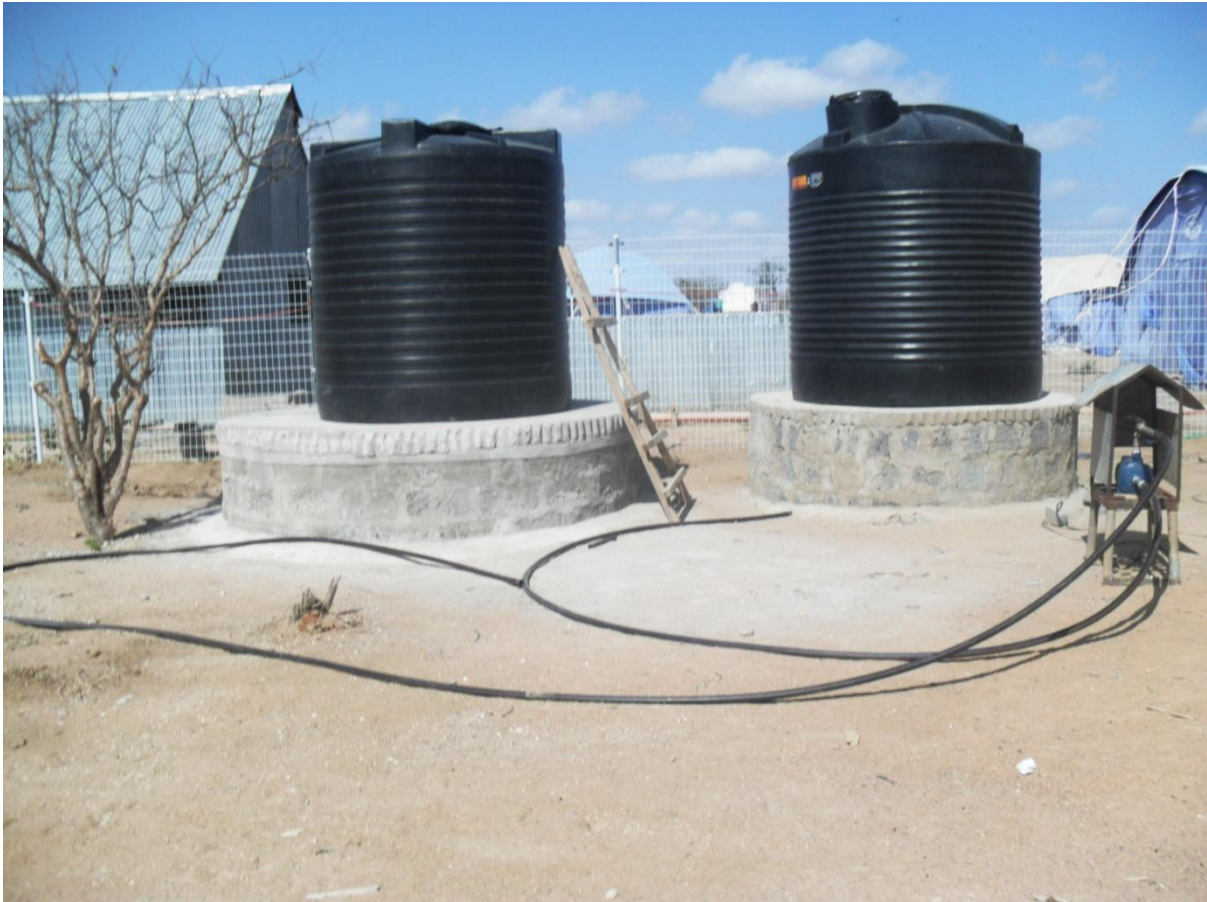
Figure 9: Water storage tanks
